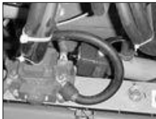
BATTERY ISOLATOR BLOCK WATER HEATER
